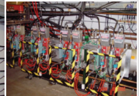
power amplifiers (TWTs)
